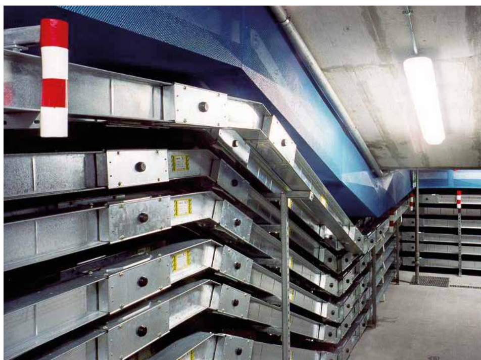
Example of high power distribution
